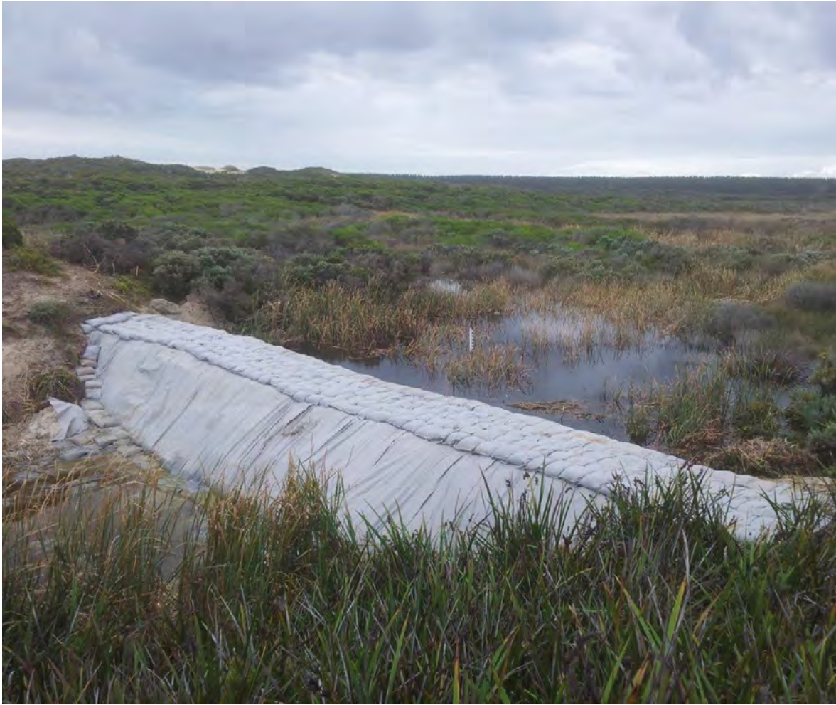
The phase 3 trial structure (foreground) has begun to regulate wetland levels in Long Swamp (background) by restricting flows from the Nobles Rocks outlet (© Copyright, Mark Bachmann)
