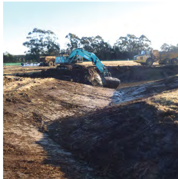
Construction of the NCIG green and golden bell frog habitat (© Copyright, Michael Godschalk, NCIG)
